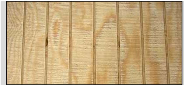
Above: Weak and fragile building materials do not adequately withstand the elements and quickly deteriorate leaving an unsightly appearance
