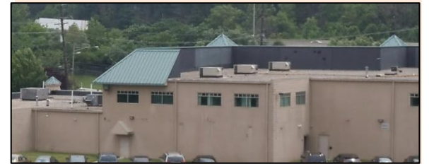
Above: Stage set roof types are an effective means to screen rooftop mechanical equipment.
